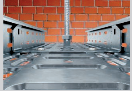
Securing of the threaded rod on the centre suspension with additional hexagonal nut.
