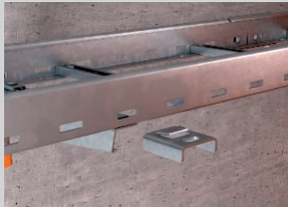
Attachment of the connection component on the lower flange of the ladder rail.
