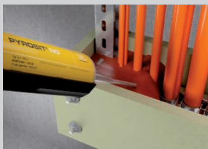
Filling of the complete housing with high cable assignments with PYROSIT® NG fire protection foam.
