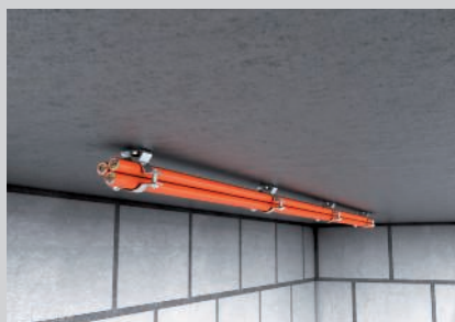
Bundled cable routing under the ceiling.
