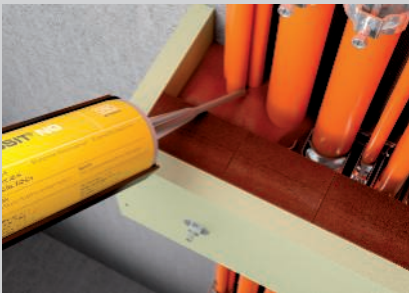
Filling with PYROPLUG® Block foam blocks and filling of the cable spandrels with PYROSIT® NG fire protection foam.
