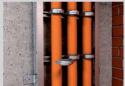
Cable installation with clamp clips on the rungs of the vertical ladder.
