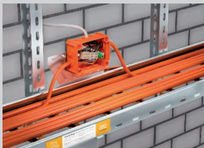
FireBox with mounting plate, type B, mounted to the rear of a cable ladder.
