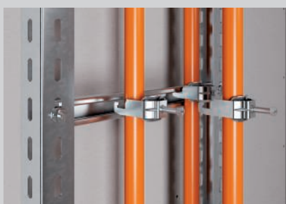
Cable installation with 2056 UM clamp clips on the rungs of the vertical ladder.
