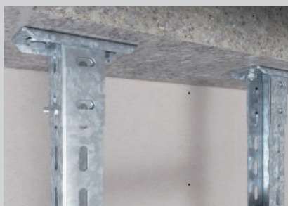
Ceiling fastening of the ladder rails with screwed-on head plates.
