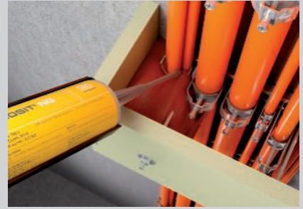
Filling of the complete housing with high cable assignments with PYROSIT® NG fire protection foam.
